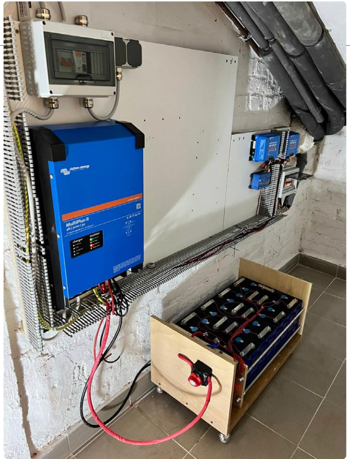
Figure 7: The complete solar battery system installed in the cellar (Source: Martin Jepkens).
